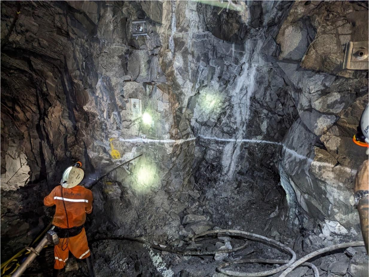
Figure 1. Photo of the first cut on the lode, strike drive from the new development decline.
